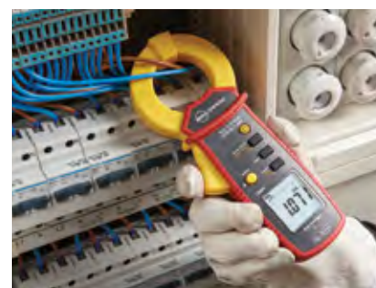
Differential current measurement with leakage current clamp
